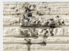
Dirt is attached to the surface.
